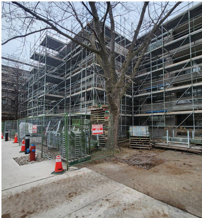
Hillside Place is a seniors' residential building that is part of a community energy project funded by the CCBF that will see the current natural gas heating system replaced with an energy-friendly heat pump system, providing both heat and air conditioning to the building.
